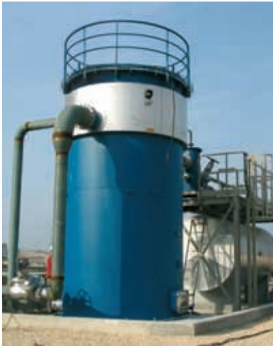
SEREP DEOILER DE 27 deballasting plant
